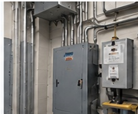
03. Back room - electrical panel
